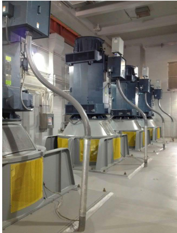
Western Flood Pumping Station motor gallery.
