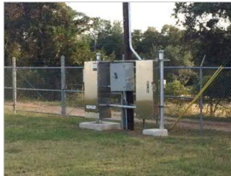
Electrical service and generator transfer switch.
