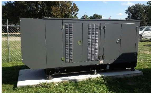
Natural gas water pumping station generator.
