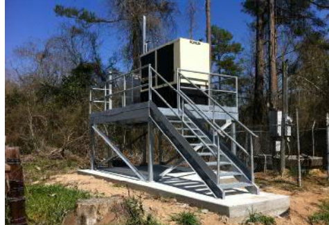
Melton Street lift station generator.
