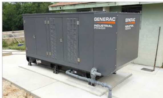
Generator at wastewater treatment plant.
