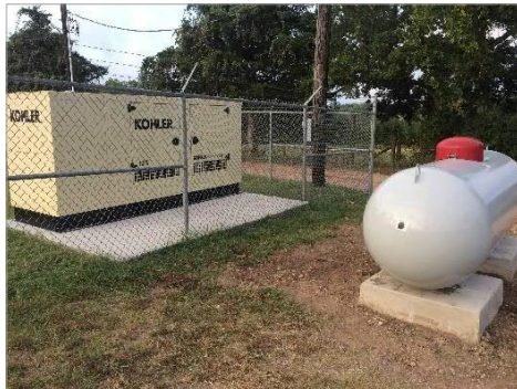
Round Top water plant generator.
