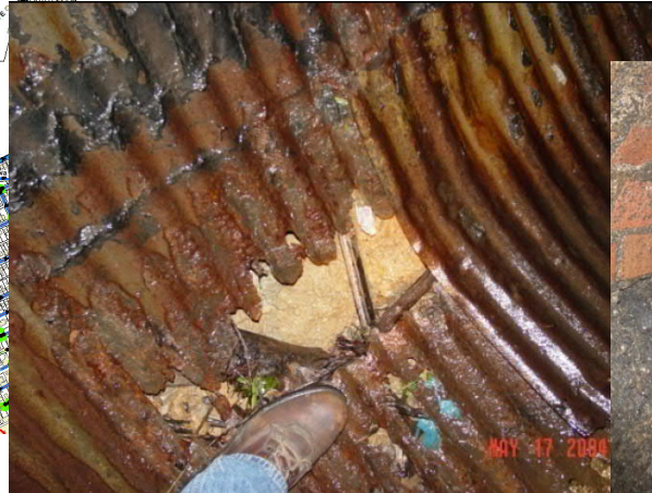
Corroded CMP Culvert
