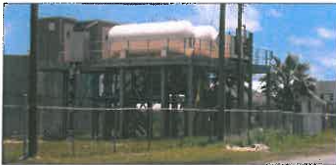
Treasure Island MUD Elevated Water Plant
