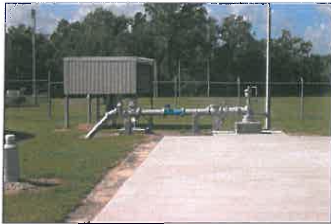
Galveston County WCID No. 8 Water Well
