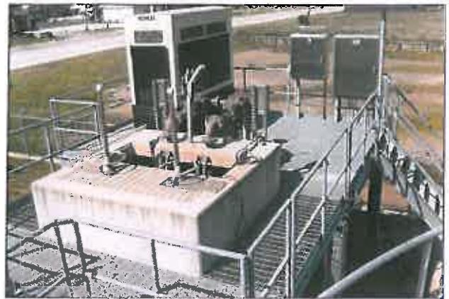
Galveston County FWSD No. 6 WWTP Lift Station
